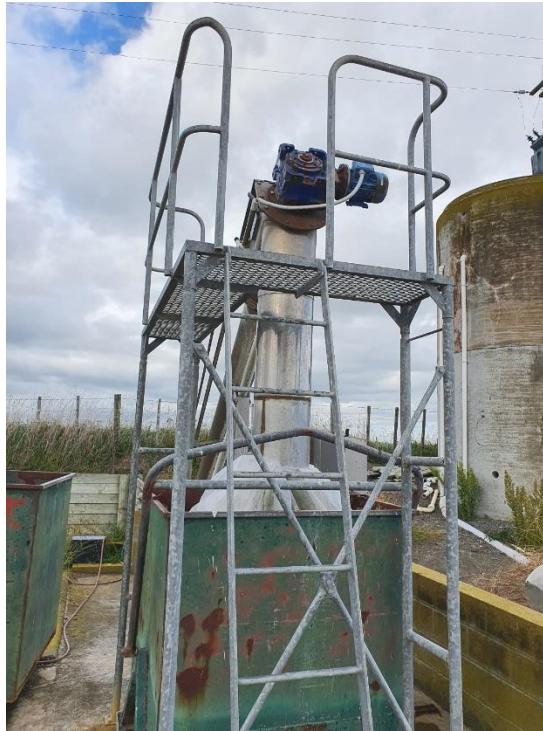
Figure 5-2: Ratana WWTP inlet Screen handling system
