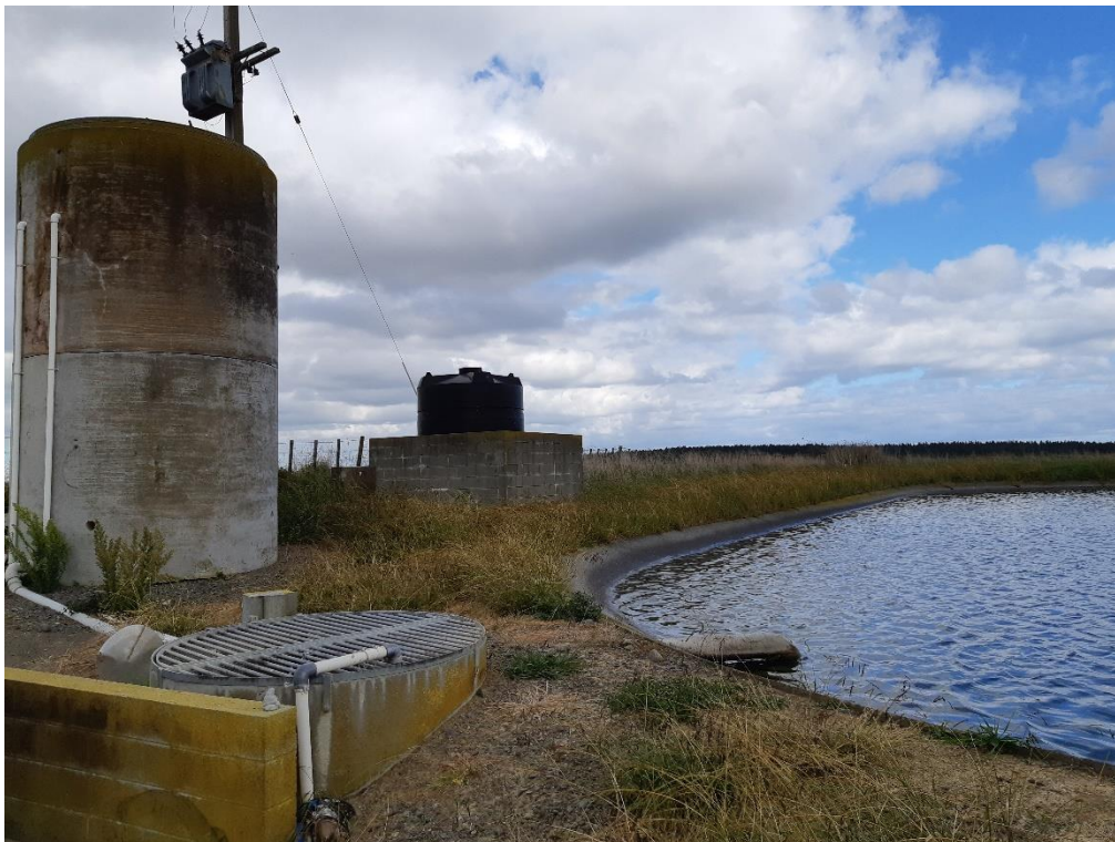
Figure 5-3: Ratana WWTP Biotower and Pond 1 inlet
