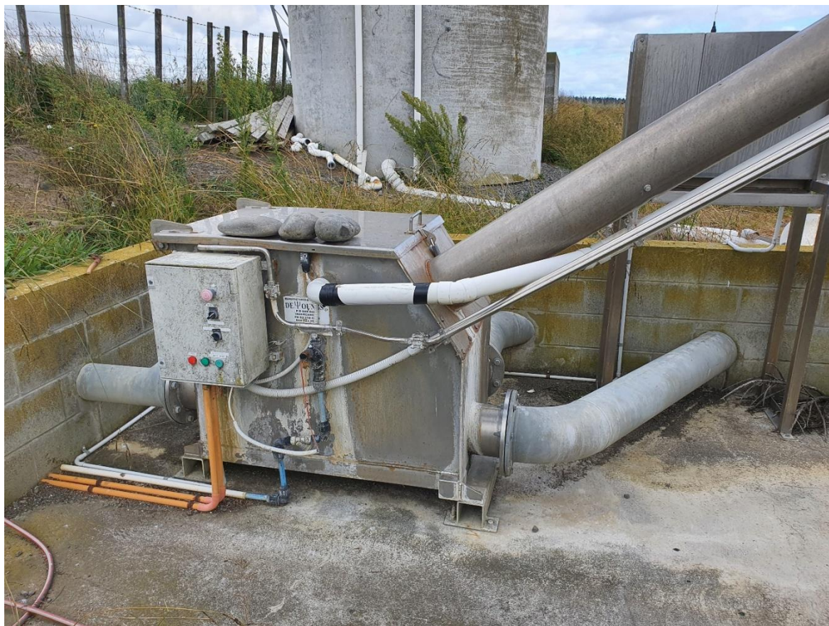
Figure 5-1: Ratana WWTP inlet Screen
